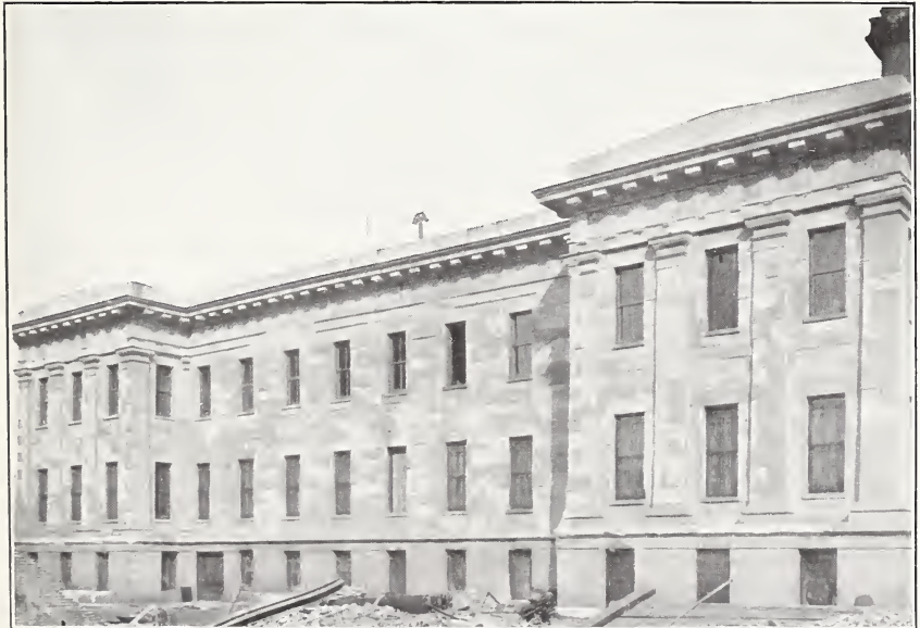
B. SPALLING OF STONWORK BY FIRE, NORTHWEST FRONT OF UNITED STATES MINT.
